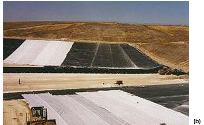
FIGURE 23.14 (a) Idealized diagram of a solid-waste facility (sanitary landfill) illustrating multiple-barrier design, monitoring system, and leachate collection system. (b) Rock Creek landfill under construction in Calaveras County, California. This municipal solid-waste landfill is underlain by a compacted clay liner, exposed in the center left portion of the photograph. The darker slopes, covered with gravel piles, overlie the compacted clay layer. These form a vapor barrier designed to keep moisture in the clay so it won't crack. Trenches at the bottom of the landfill are lined with plastic and are part of the leachate collection system for the landfill. The landfill is also equipped with a system to monitor the water below the leachate collection system.
