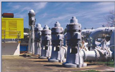
Public supply water intake, Bay County, Florida
